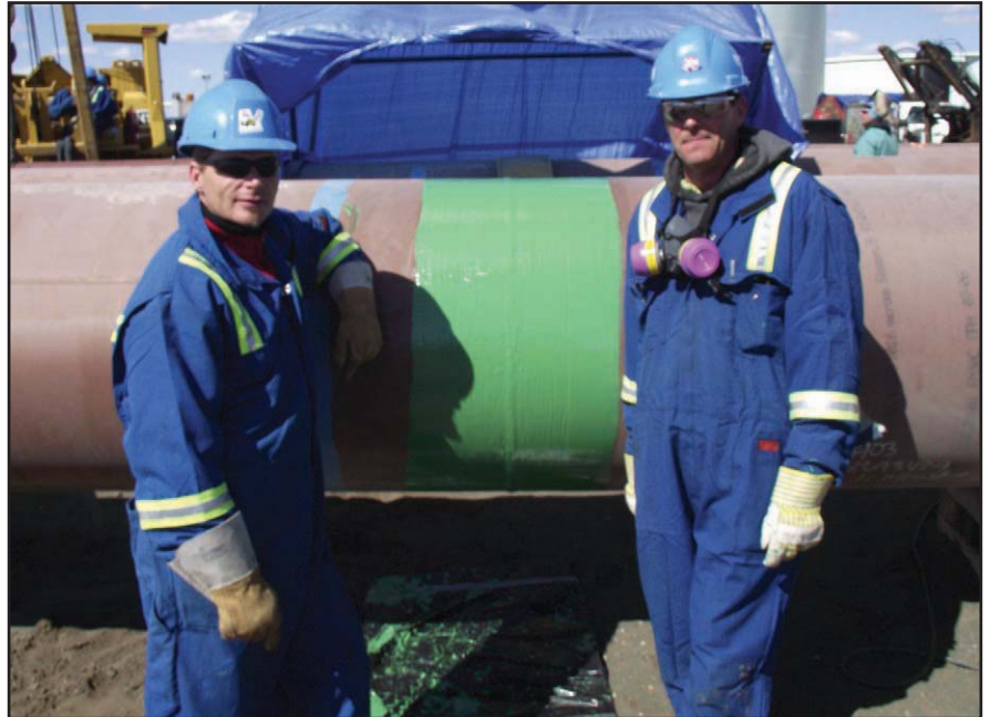
The highly skilled crew from Ledcor with a recently completed a Protal 7200 protected joint.
