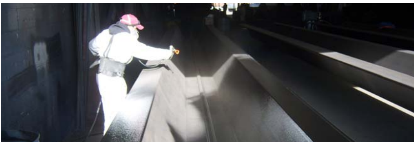
Denso Rigspray being applied to steel sheet piles with an airless spray unit.
