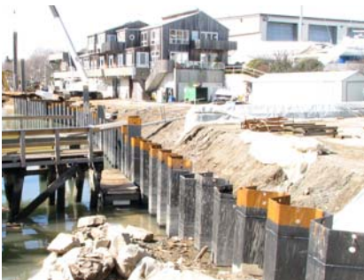
Side view showing initial phase of the Boston Marina using Denso Rigspray steel sheet piles.
