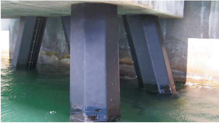
SeaShield Series 2000HD System was used to protect octagonal concrete bridge piles.
