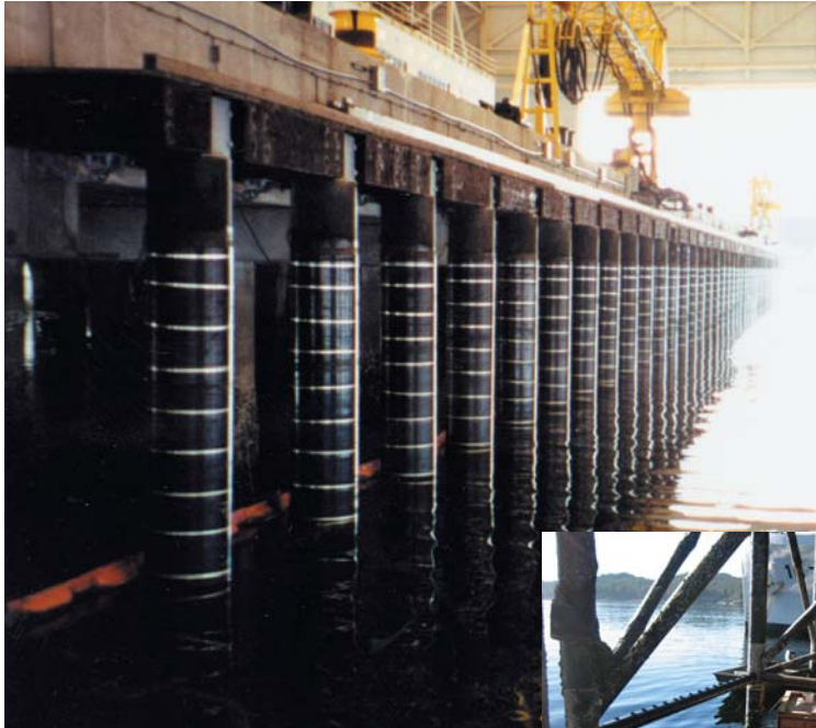
The U.S. Navy installed the SeaShield Series 100 System to protect over 400 ea. 24" to 30" steel piles.
