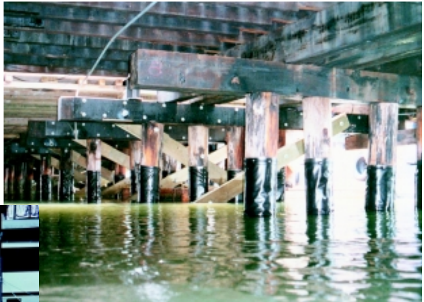
The Series 30 System was used to protect timber piles at the Fort Monroe Naval Facility.
