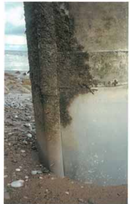
Close-up of 850mm diameter pile illustrating raised beach level and marine growth in 1995.
