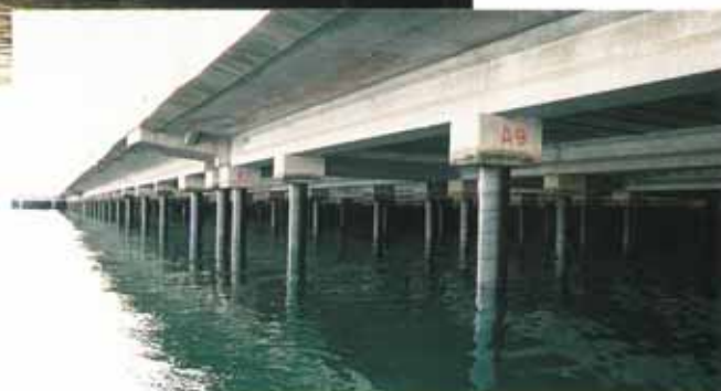
SeaShield protected piles supporting the runway.
