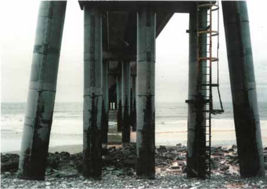
View of system 3-4 years after installation.
