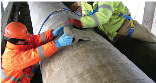
Denso LT Tape was applied in a short amount of time to concrete pipe, providing reliable protection.
