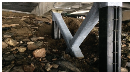
Steel cross beams protected with Denso Glass Outerwrap UV in lieu of the 80 mil HDPE Outercoaters.
