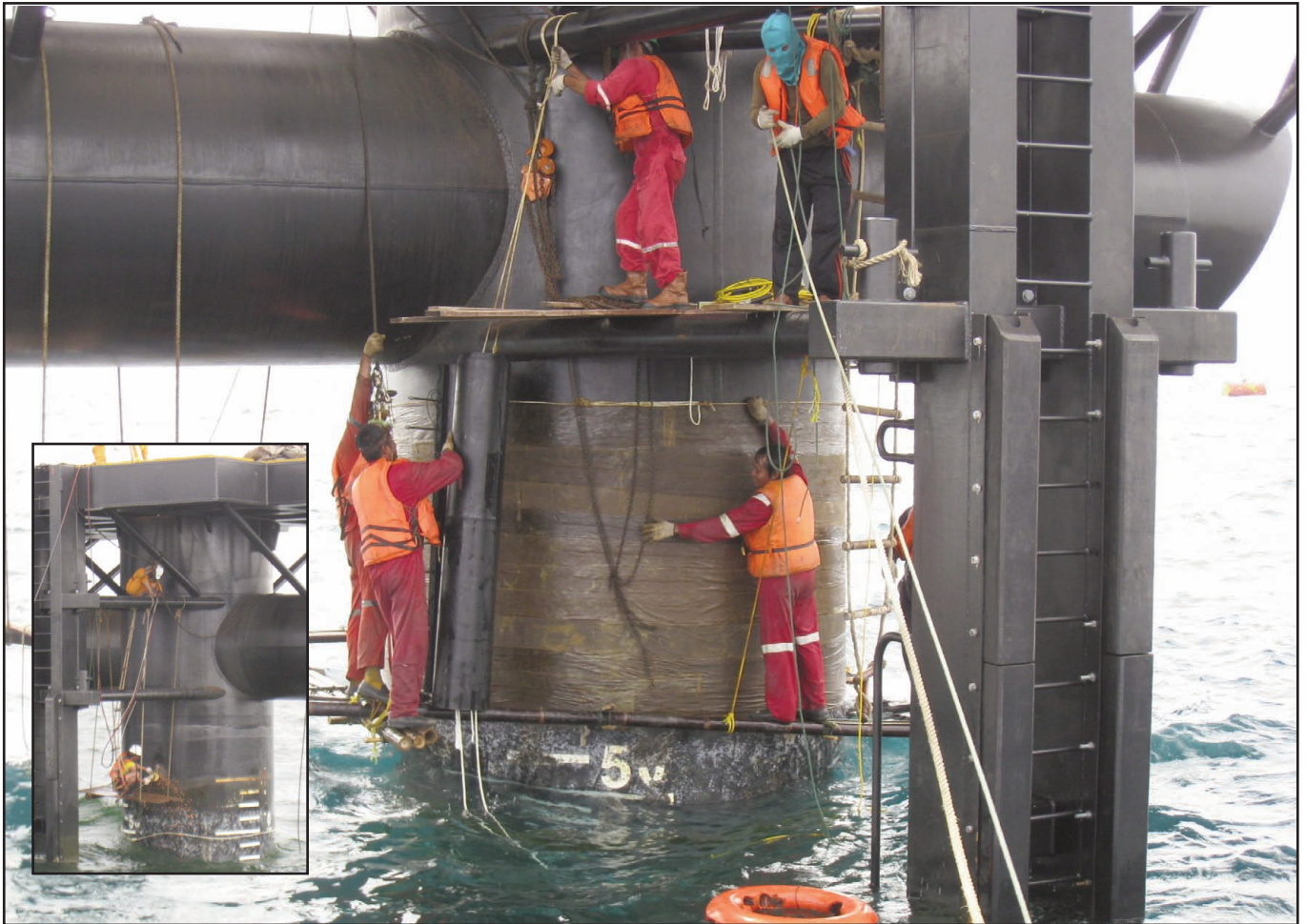
After first cleaning the designated pile area (inset) for the SeaShield system, a coating of Denso S105 Paste is followed by a double wrap Denso Marine Piling Tape.
