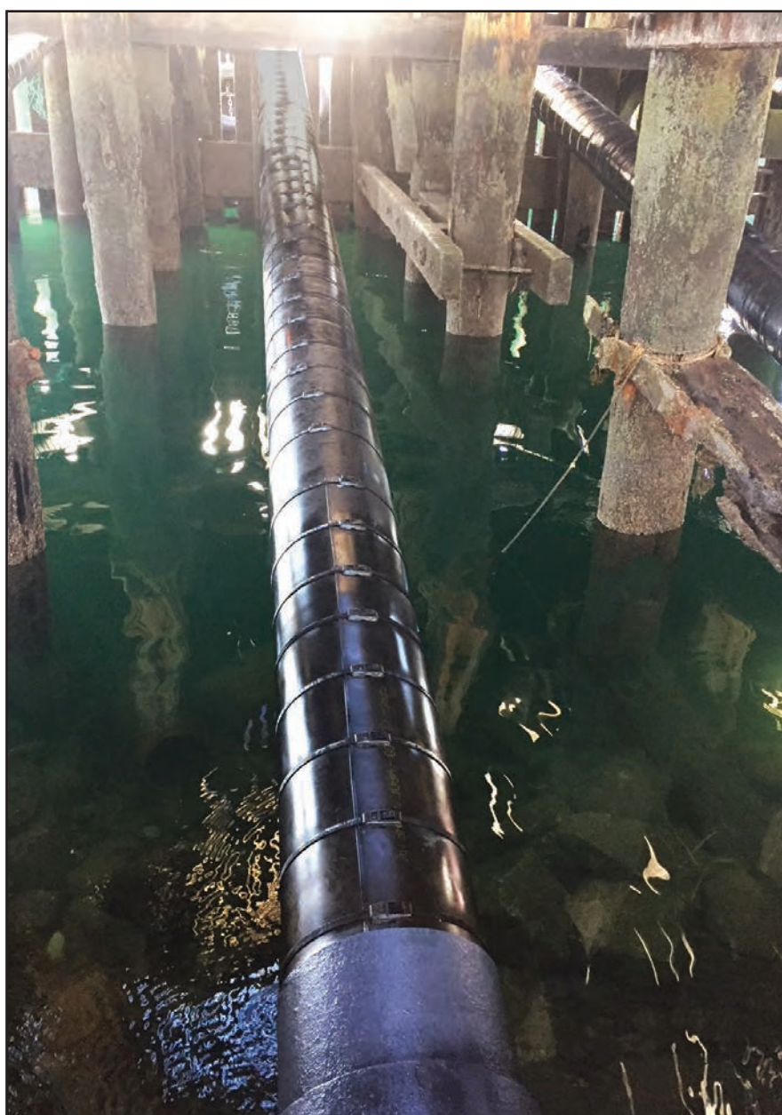
Pipes under the old pier protected with SeaShield 100™.
