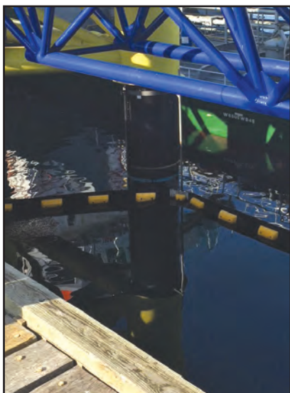
One of the jetty piles on the new pier protected with SeaShield 2000 FD™.
