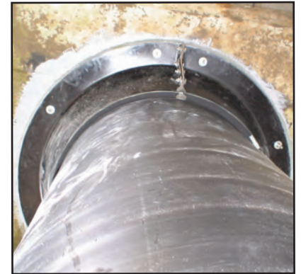
Close up of the seal between the Denso Pile Cap and concrete jetty soffit.
