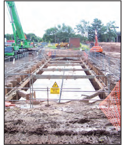
Above: The jointed culverts in position. Below: Tokstrip being applied to a culvert joint face
