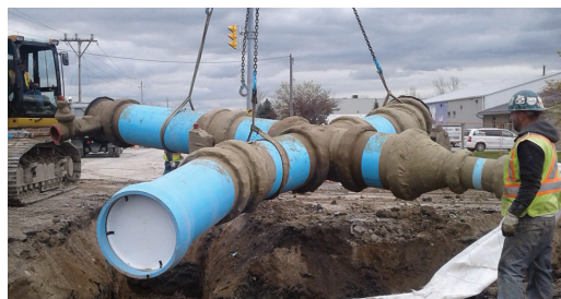
Fully corrosion protected valves using Denso Petrolatum tape being lowered for buried installation.
