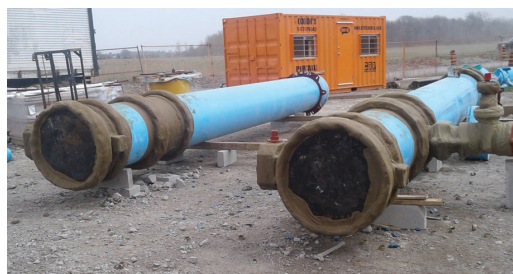
Some of the Denso Petrolatum Tape System installation was applied prior to placing in-situ.
