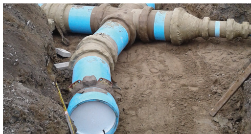
Metal valve assemblies and fittings protected with the Denso Petrolatum Tape System.
