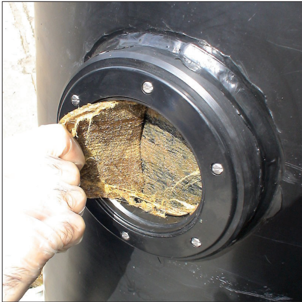
With the cover removed the petrolatum tape layer can be cut back to expose the pile surface for inspection.
