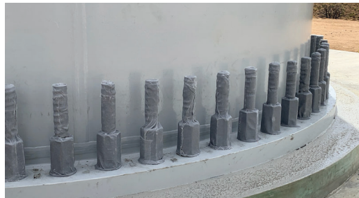
Over 900 windmill anchor bolts were protected from environmental corrosion with Denso ColorTape.
