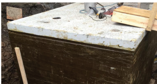
Hi-Tack Paste and Tape applied to the entirety of the structure to prevent water ingress and infiltration.
