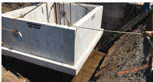
Chamber being set on pre-laid Hi-Tack Tape strips for waterproofing of the base.
