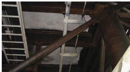
Denso Hi-Tack Tape after 8 years service life.
