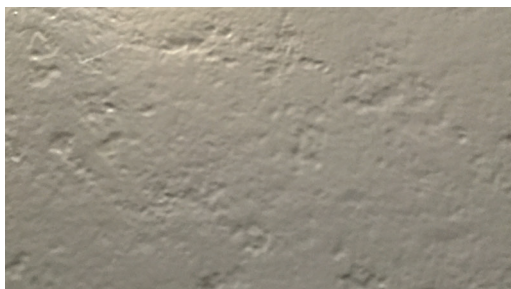
Heavy pitted floor with 401/476 pinhole free.
