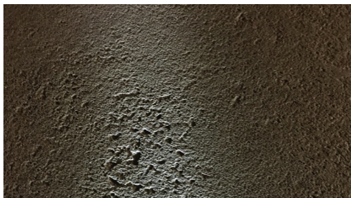
Heavy pitted floor.
