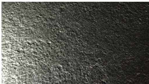
Heavy pitted floor with 401 sealer.
