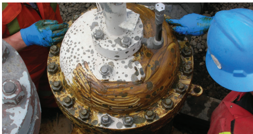
Denso Paste used to prime surface to displace moisture and penetrate rust before applying mastic and tape.
