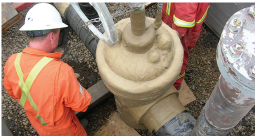
A final wrap of Denso LT Petrolatum tape to finish the job - note the flexibility of the tape and ease of wrapping over awkward shapes.
