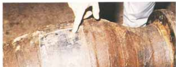
The petrolatum compound (brown) still adheres to the black metal substrate.
