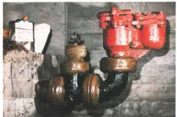
Denso materials have been used in 13 valve chambers.
