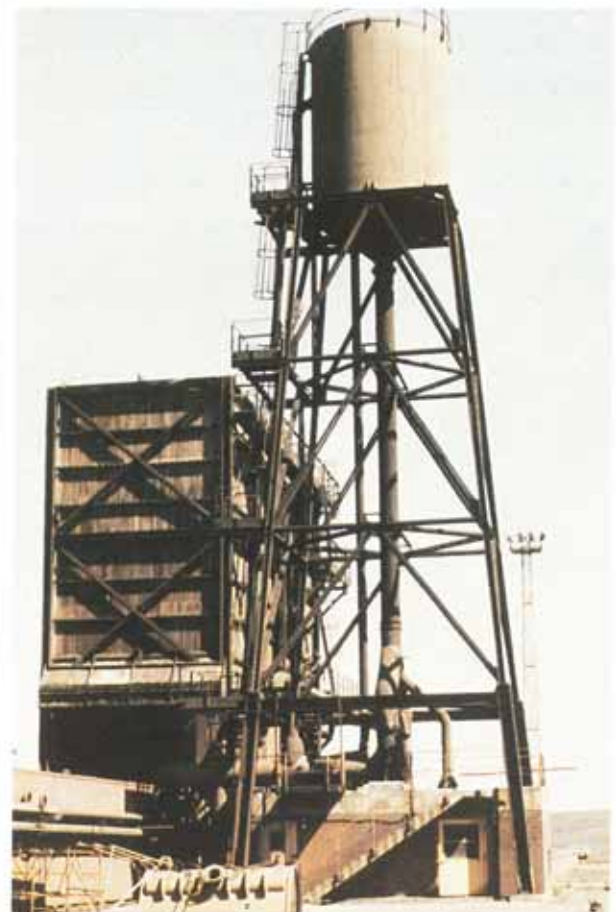
Water tower and quenching station at coke oven battery under Denso wrap.
