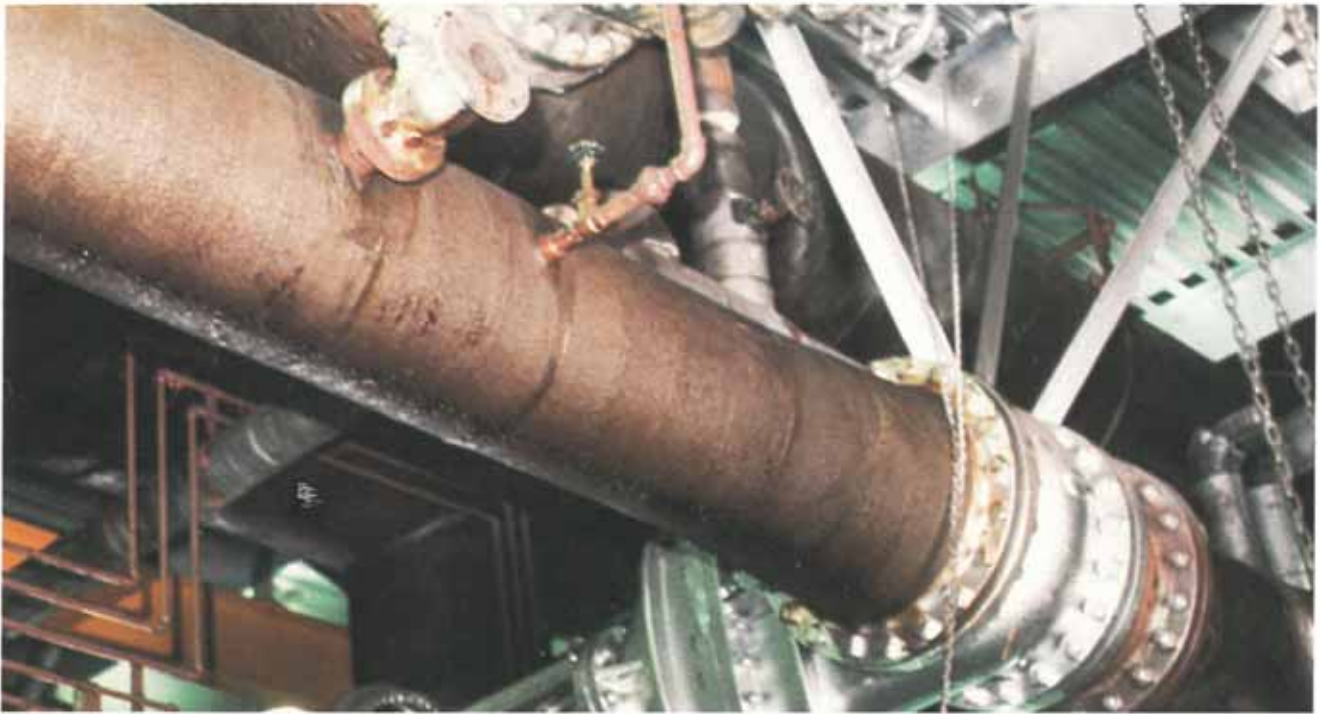
Water lines at blast furnace pump house.
