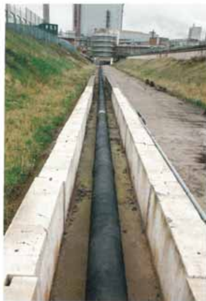
Pipeline protected by the Denso Covercoat System.
