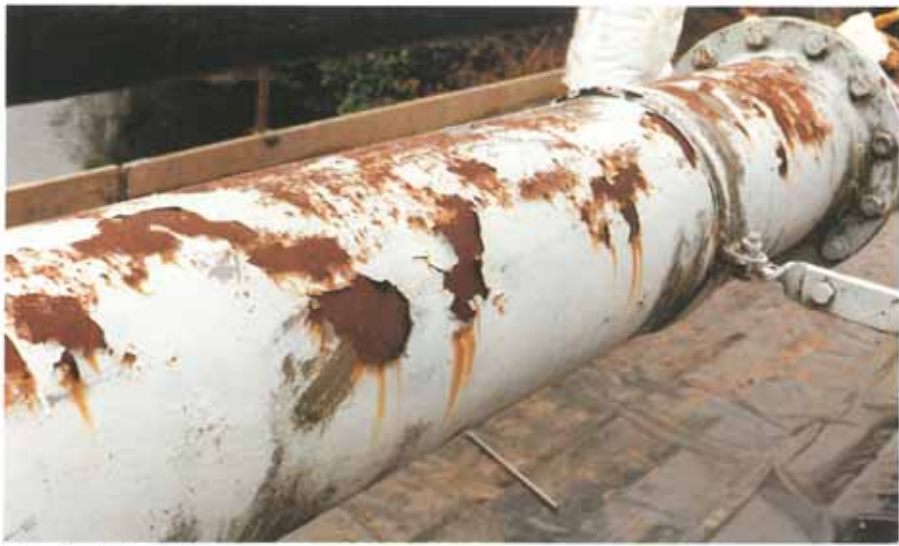
The deteriorated original coating.
