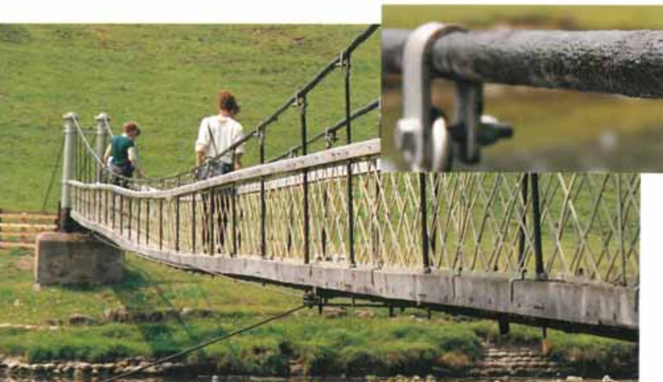
The suspension bridge with Denso Covercoat armoured cables.
