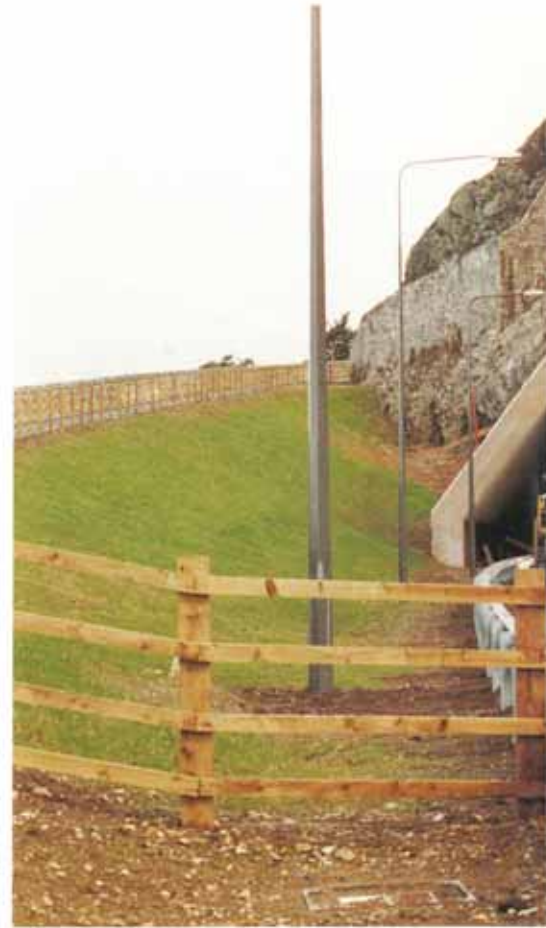
The tunnel entrance showing ground anchors featured in a previous Denso Digest.
