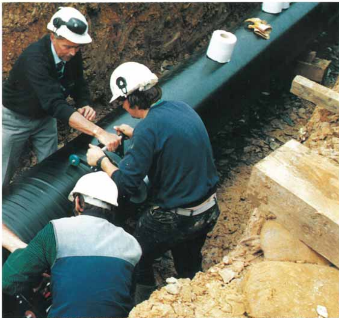
The use of two Demosem Wrapping Machines in tandem speeded up the application of the Demoseal 70 Tape.
