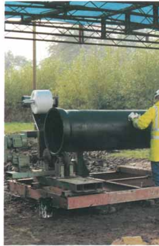
Each pipelength is primed with Demo Primer D and the surface is checked for defects and retouched if necessary before wrapping commences.
