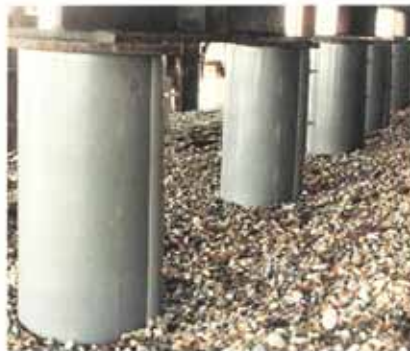
Series 200 System half buried in shingle.
