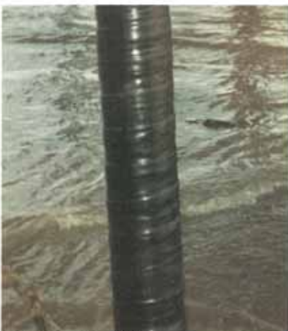
Series 80 System installed 1982.
