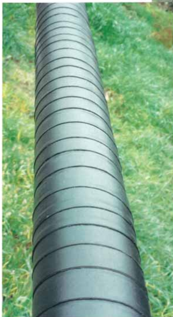
Close up of machine wrapped pipe.
