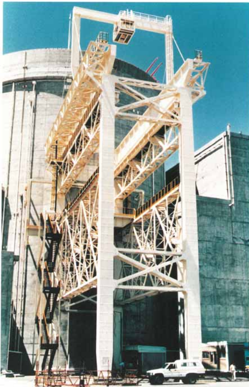
One of the two huge cranes based at a Nuclear Power Station in The Cape fully coated with the Fire Resistant Denso Covercoat System, which has a service life six times greater than conventional heavy duty paint systems applied to wire brushed steel surfaces. The crane project involved 12,000 m 2 of Covercoat and was selected by the S.A. Corrosion Institute as one of the top three outstanding coating contracts of the year.
