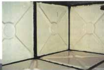
A second stripe coat is applied after the application of the intermediate (cream) coat.
