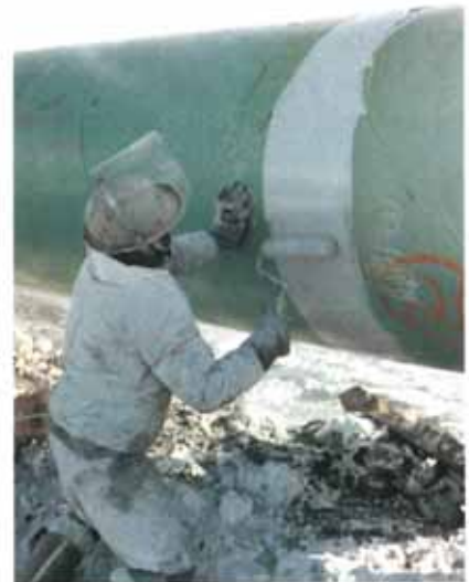
Protal 5900 being applied by roller to 1.06m (42") girth weld in -28°C (-20°F) winter conditions.
