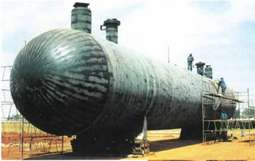
Densotherm 30 Coating being applied to mounded LPG Storage Vessels for the Afrrox Project in the Transvaal.
