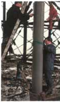
Series 200 System installation December 1984.
