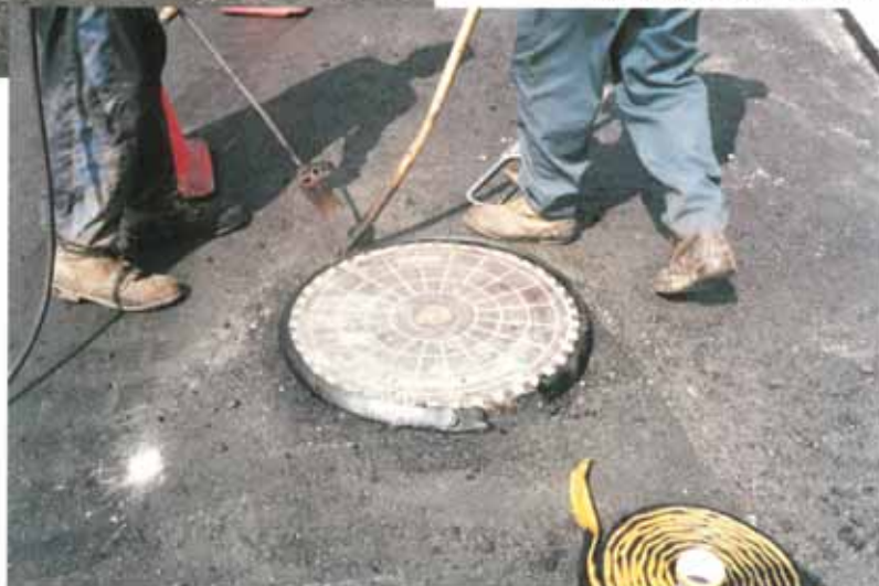
Tokband Spezial used to form a flexible seal between an iron manhole cover and the asphalt wearing course.
