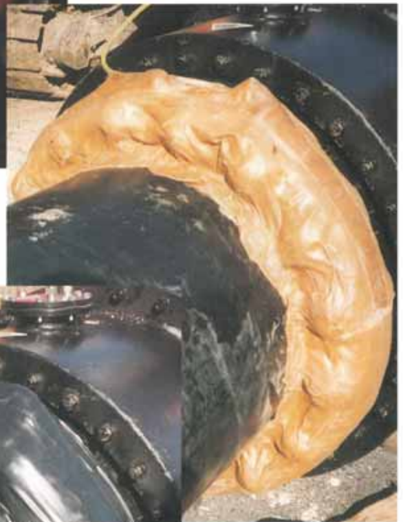
The Denso Mastic and Denso Tape have been applied to the flange assembly.
