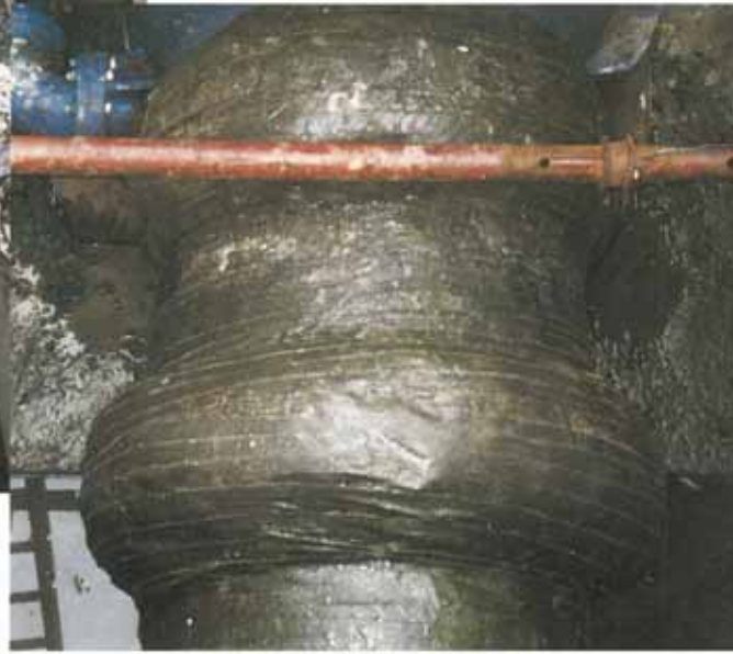
A protected flange joint.
