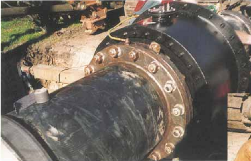
The magnetic flowmeter is shown connected to a new pipe main and the nut/bolt assemblies protected with Denso MP Primer.
