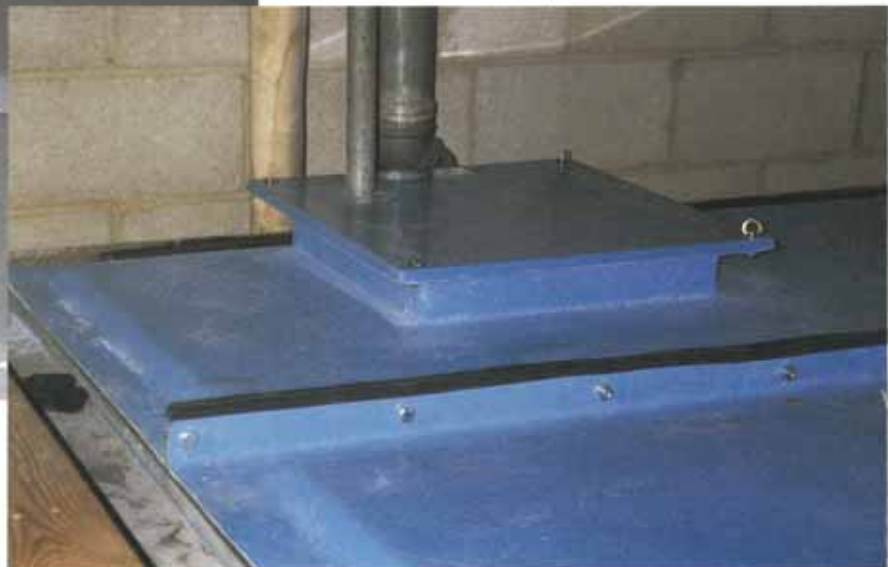
Nu-Lid 30 water tank lid in position.
