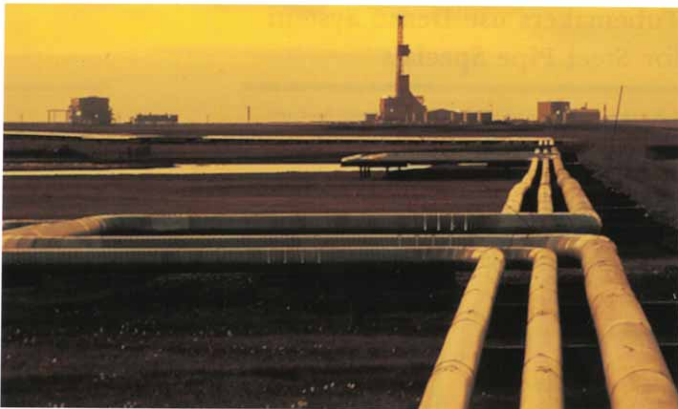
Above ground oilfield pipelines, The North Slope of Alaska.
