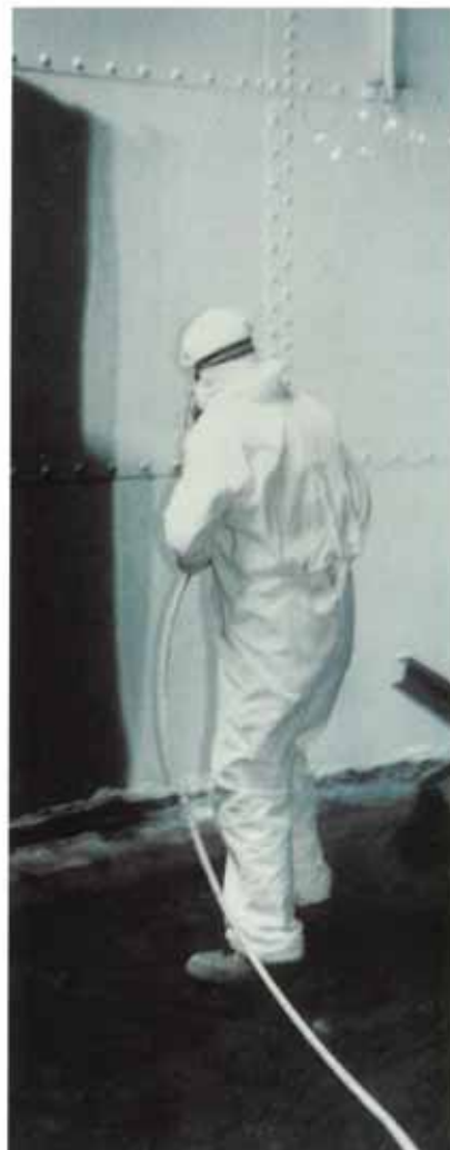
Spray application of Archco-Rigidon 423D glass flake filled vinyl ester resin coating.
