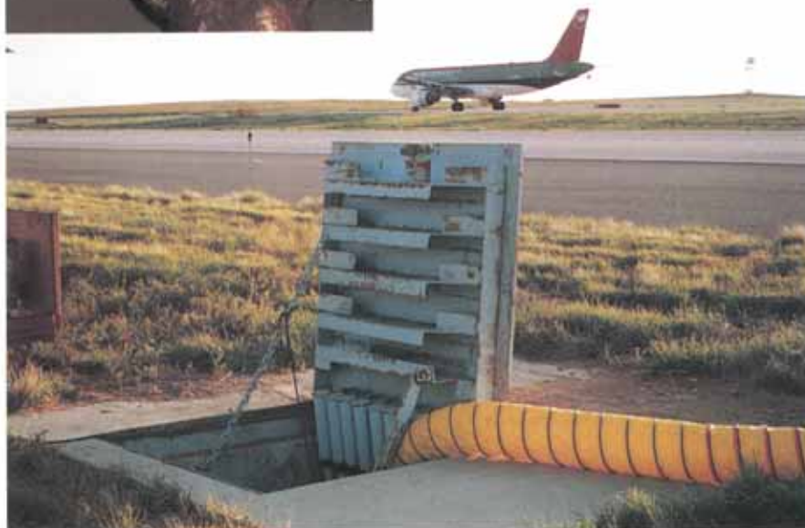
Below: One of the 204 vaults in close proximity to the airport runway.
