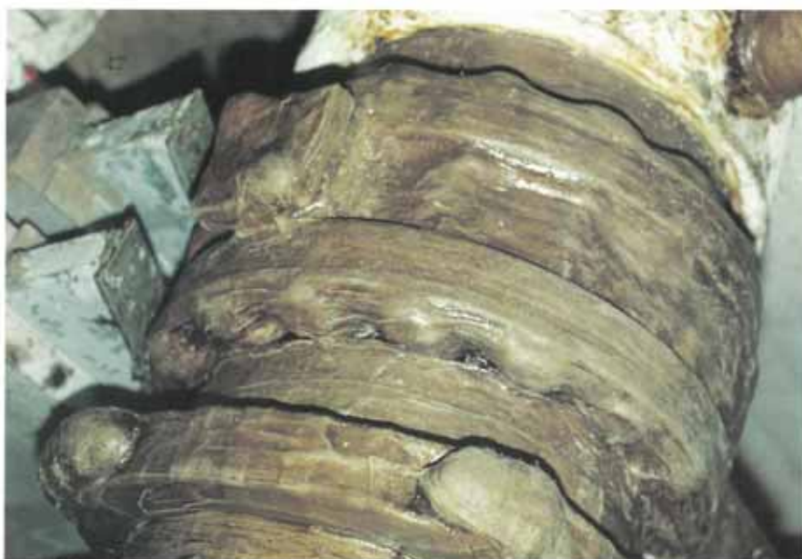
A joint is wrapped with Denso LT Tape to complete the protective system.
