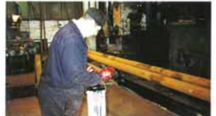
Denso Primer D is applied to cleaned surface and allowed to dry.
