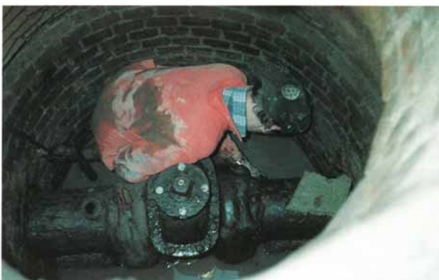
Application of Denso Profiling Mastic smooths the joint profiles prior to wrapping with tape.
