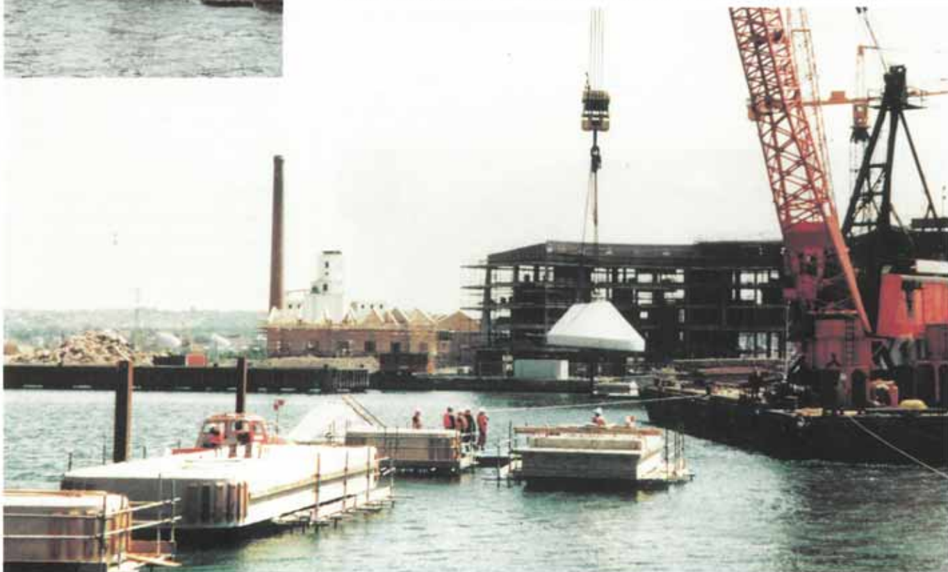
Tokstrip was applied to the cone-shaped bridge supports before they were lowered into position on the tubular piles.
