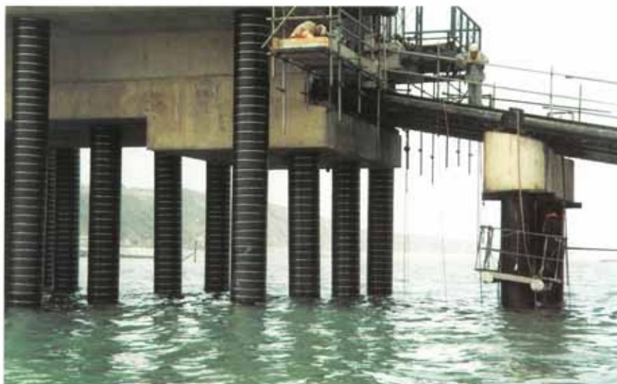
Left and above: View of the new lifeboat house and slipway piles showing the installation of the SeaShield 100 System in progress from suspended platforms.
