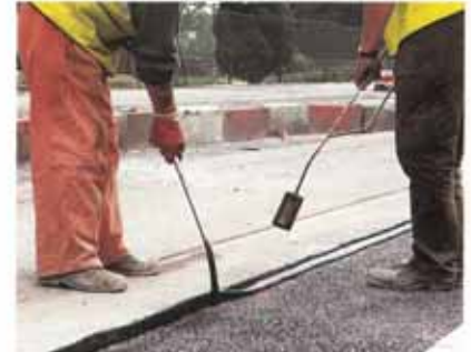
Densoband is applied to the joint face prior to laying the new asphalt wearing course.
