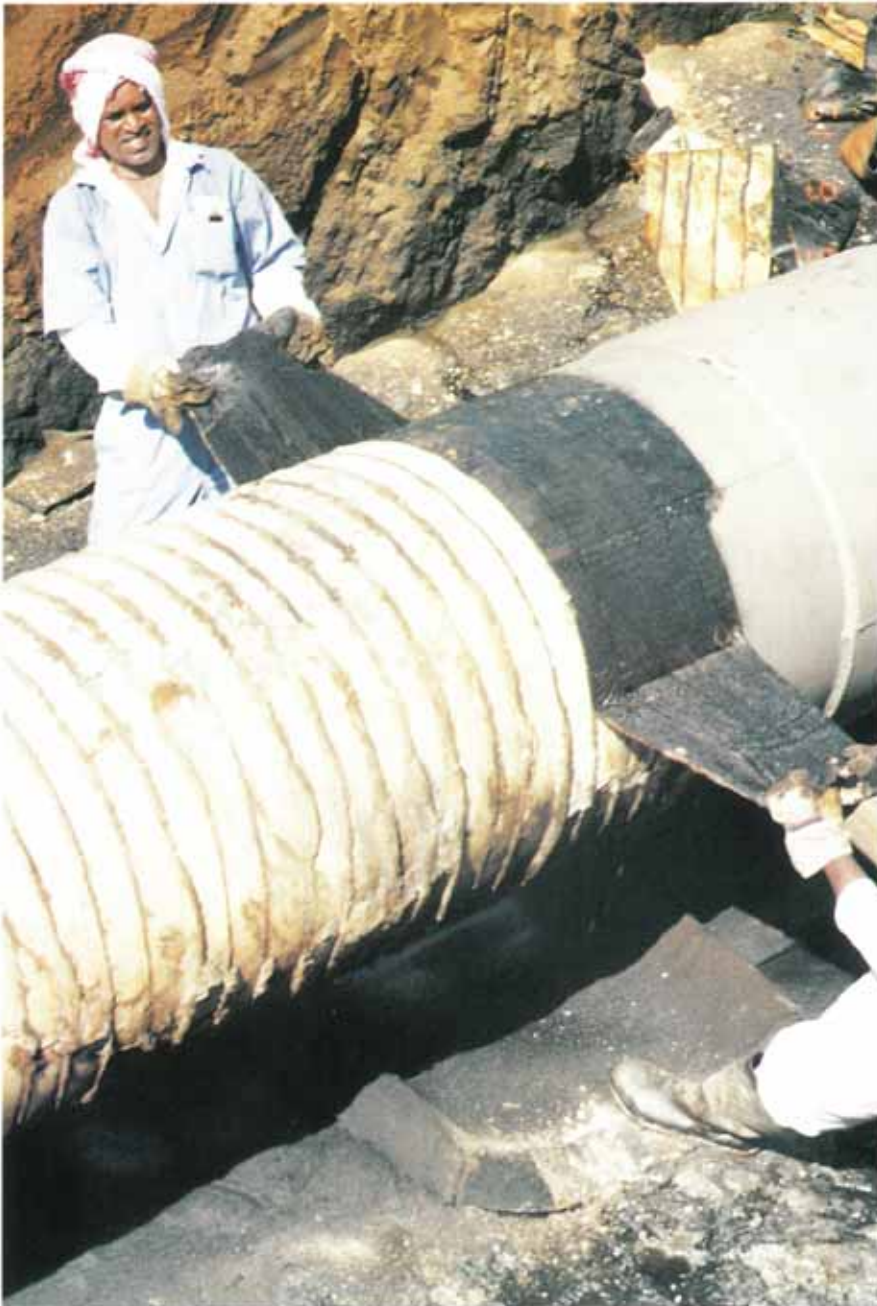
Inspection of the pipeline involved removal of the Densopol 80 HT Tape after 14 years burial in highly corrosive soil conditions.
