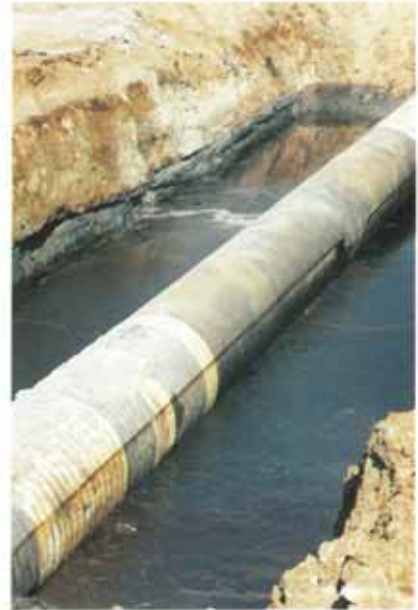
Excessive ground water mixed with the high salt deposits of this region make the conditions very demanding for the Denso corrosion protection coating.
