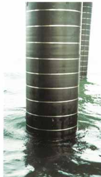
Close up of SeaShield 100 System protected pile showing stainless steel banding in place.
