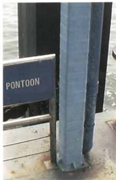
Surface tolerant and highly corrosion resistant, Denso ColourTape was spirally applied to the ferry terminal steel roof supports.
