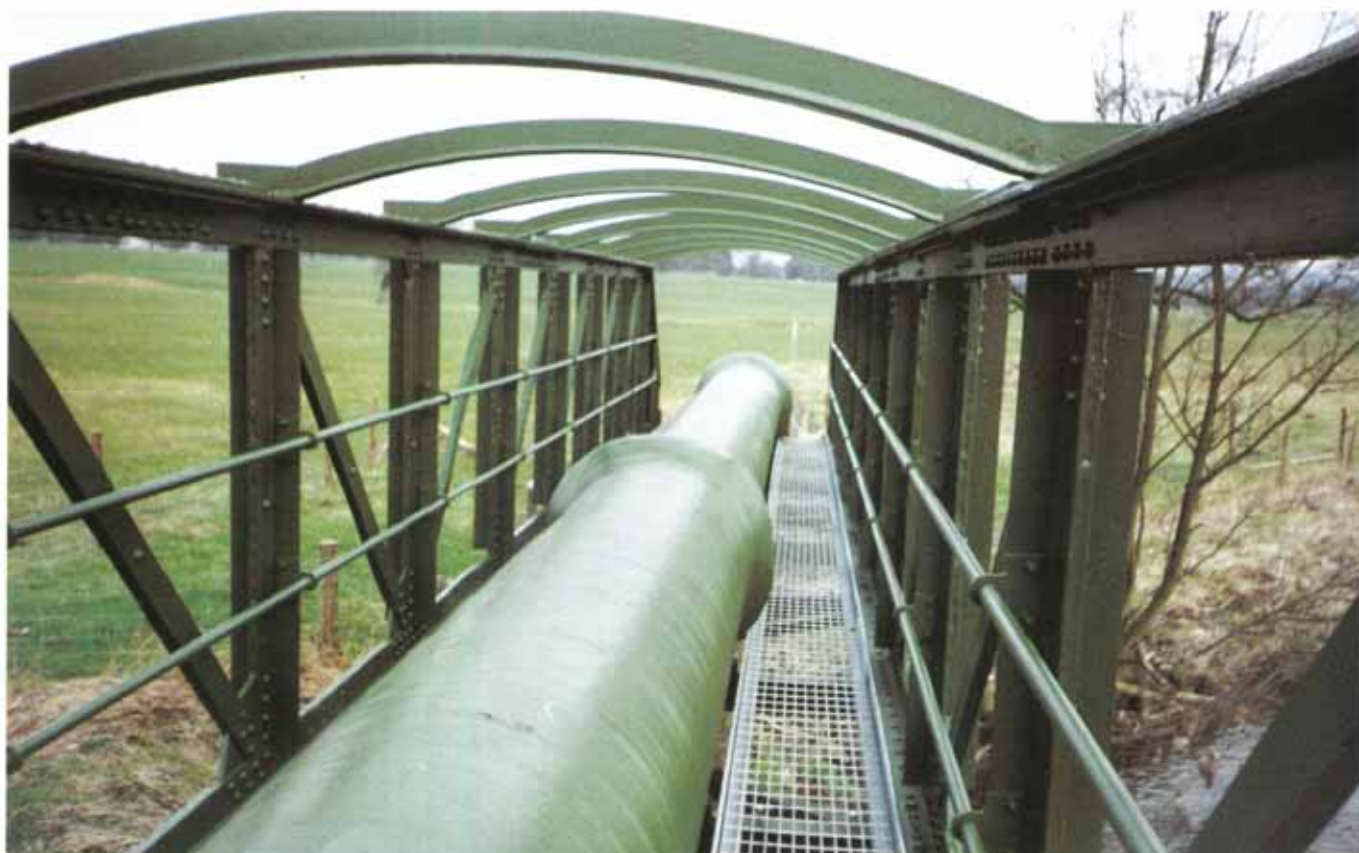
Top: Water main over the Loud Way river during application of Denso Steelcoat 400 System.
