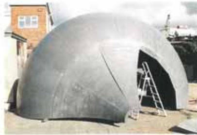
Above: The segments were joined together similar to the construction of an orange.
