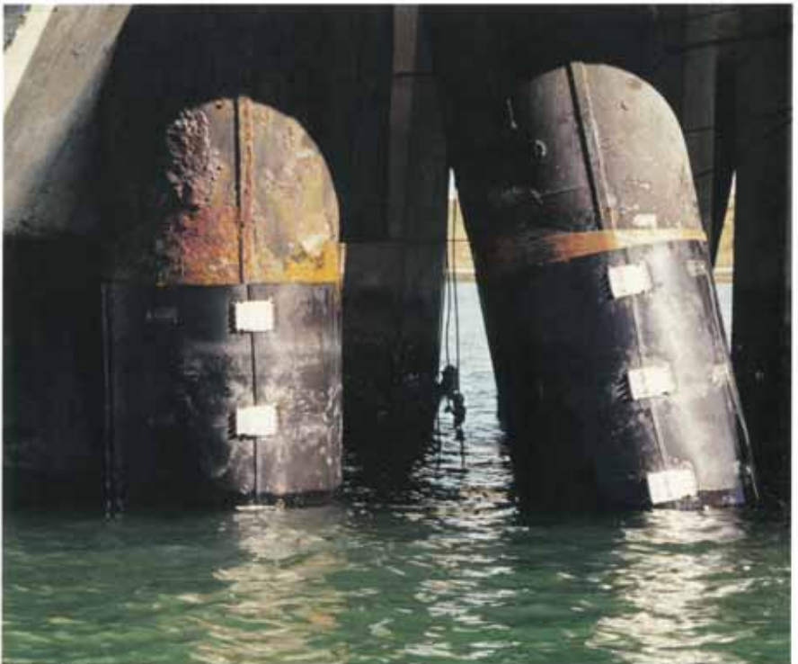
The completed SeaShield system in service.
