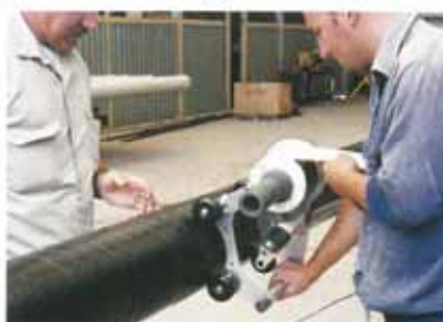
The Densoman wrapping machine speeding up the application of Denso Ultraflex 1500 System.
