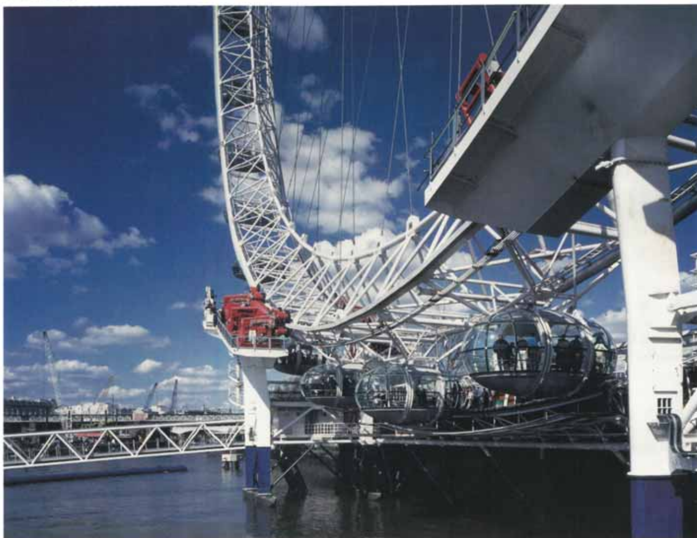
The base of the London Eye's restraint towers are partially submerged in the River Thames at high tide.
