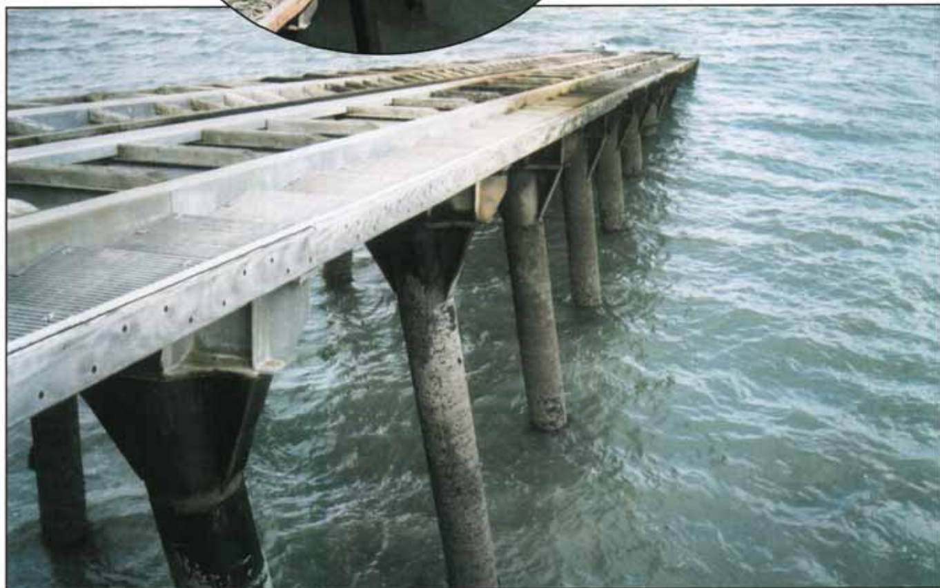
Below: February 2002 - the SeaShield protected piles.
