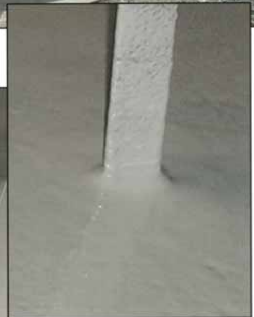
Above: Close up of the finished Denso Heatshield coating, well able to cope with the occasional vessel operating temperatures of up to 110°C.
