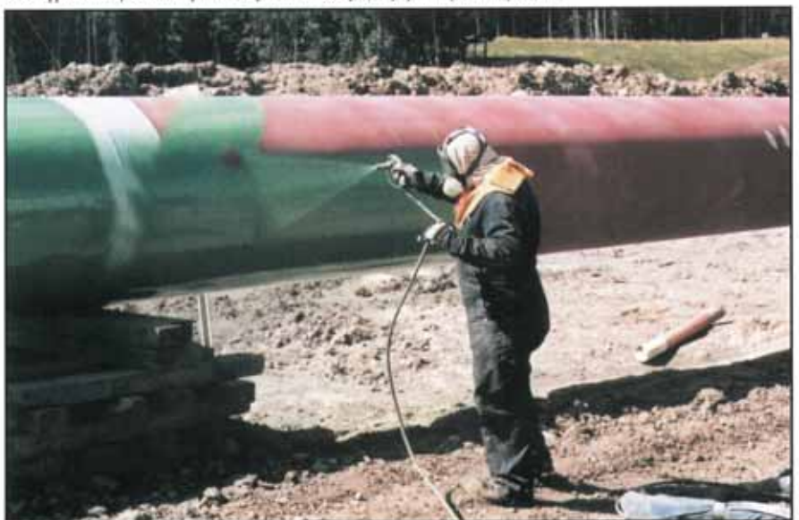
Field application by standard plural component airless spray equipment poses no problems.
