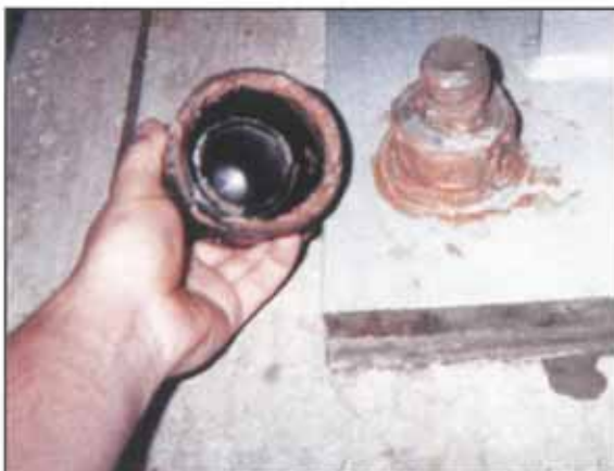
Above: Each projecting thread and nut was protected with Denso SeaShield Primer (Denso Paste S105) before receiving its Radolid cup.
