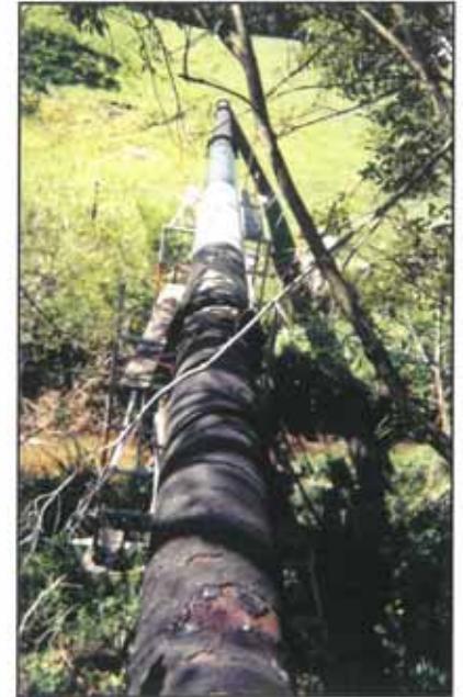
Picture foreground shows the pipe condition in some areas prior to cleaning to Swedish Standard St2.
