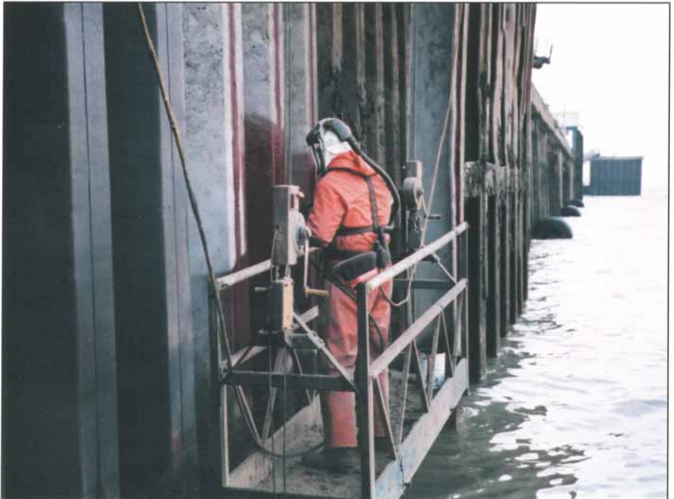
Spray application of Denso Epoxy CTR to the jetty steel sheet piling.
