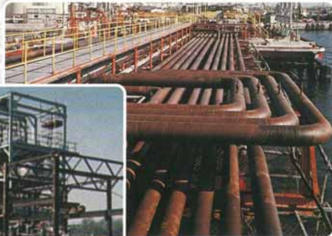
Large diameter exposed jetty pipelines protected against marine corrosion with Denso Petrolatum Tape.
