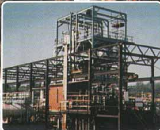
Exposed steelwork members of process plant are protected against chemical corrosion with Denso Petrolatum Tape and Acrylic Topcoat.
