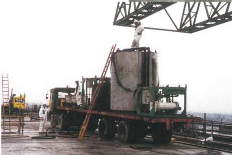
Special storage and pumping equipment, designed and built by Winn & Coales Engineering Division, in operation on site.
