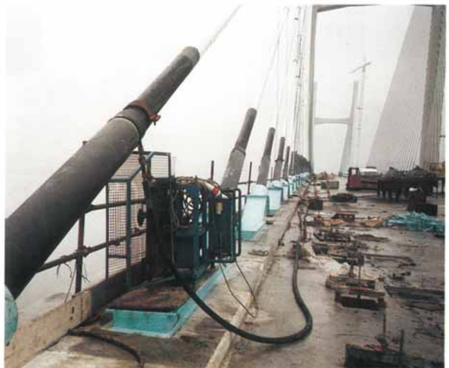
250 Metre stay cables were protected with Denso Void Filler which was pumped to a height of 100m.
