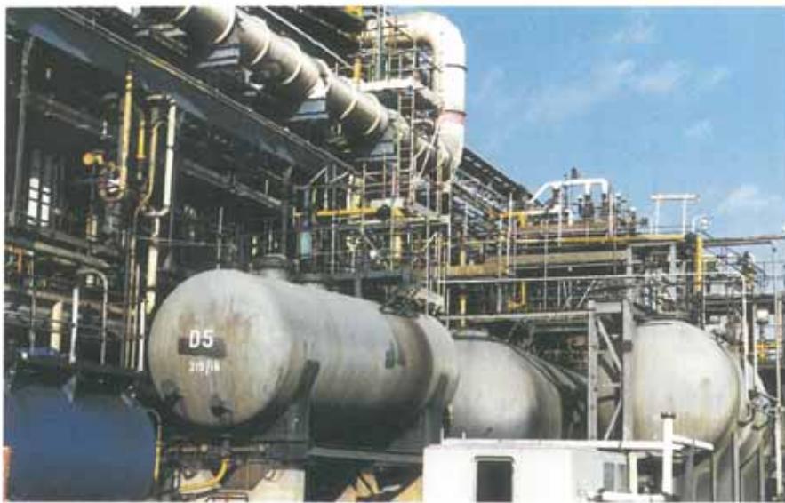
Part of Tioxides Greatham Works showing protected pipe colour coded in yellow.
