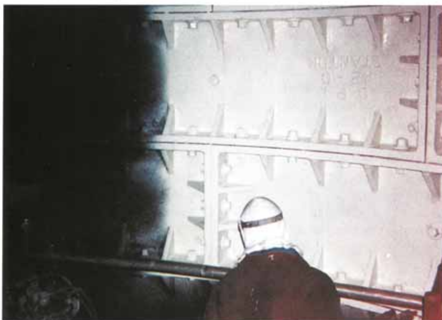
Denso S.T. Epoxy was spray applied to the bolted cast iron shaft segments.
