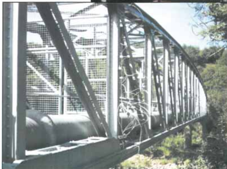
A new lease of life - the pipes were protected with the Denso Steelcoat 400/100 System and the surrounding pipebridge structure was protected with the Denso Steelcoat 700 System.
