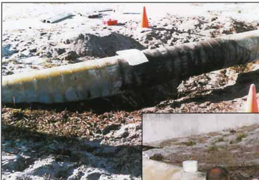
Above: Exposed pipe showing a typical fire damaged section.
