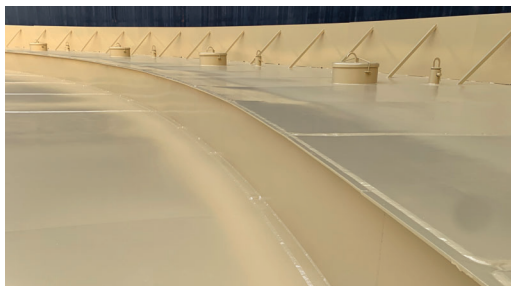
Low VOC Archco 300 Primer applied to steel tank roof prior to the application of Archco 381.
