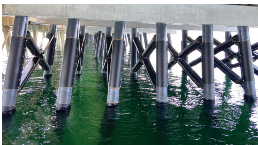
Completed Cross-Bracing fully protected with the SeaShield Series 2000HD System as well as SeaShield 525 Epoxy at node areas.
