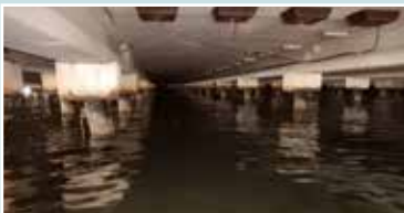
Underneath of runway showing support piles protected with a SeaShield System.
