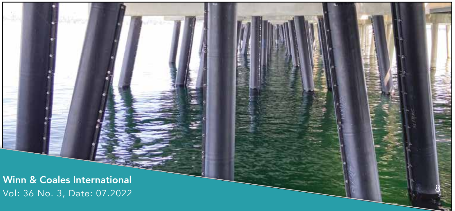
Completed 16" & 18" Dia. Cylindrical Piles fully protected with the SeaShield Series 2000HD System.
