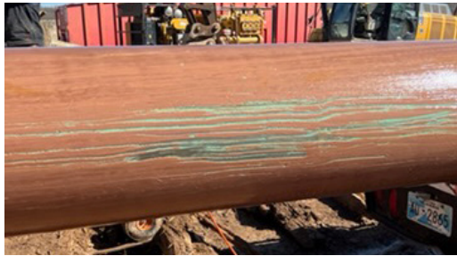
Test pull damage without a SAIG protection.
