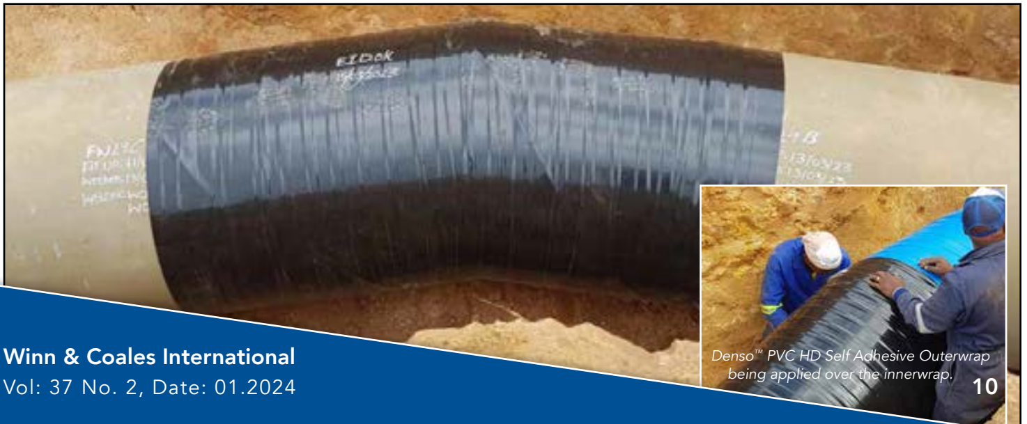
Below: Denso™ PVC HD applied at 55% overlap over the Viscowrap™ ST to offer mechanical strength and sufficient squeeze on the applied innerwrap.
