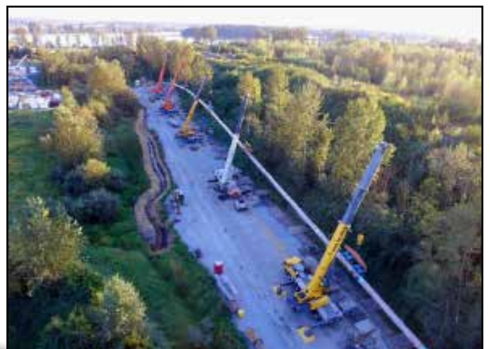
Overhead view of the installation.
