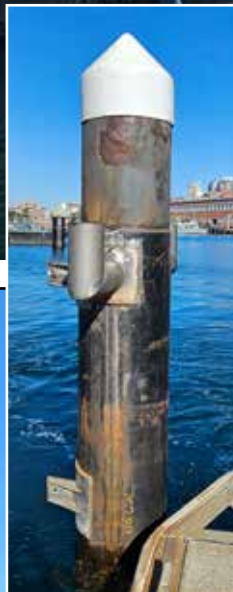
Inset: One of the piles with mooring hooks and brackets before application.
