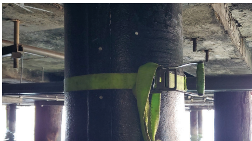
Tensionable strapping is used to hold the SeaShield™ jackets in place during injection of the epoxy grout.
