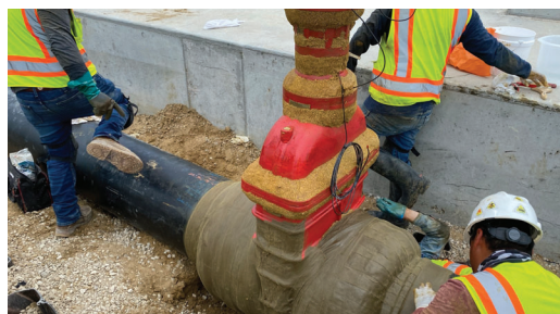
A smooth profile is achieved with Denso Profiling Mastic prior to the application of Densyl Tape.
