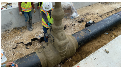
Large water valve completely encapsulated with the Denso Petrolatum Tape System will provide decades of corrosion prevention.
