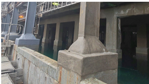
Denso Covercoat System applied to a column base before the Archco 15 topcoat is applied.
