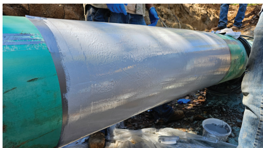
Protal 7300 Epoxy applied next as an adhesive primer for the carbon fiber system.
