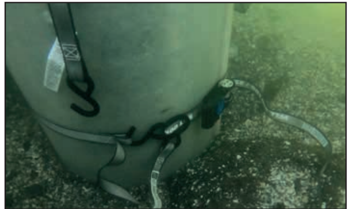
The SeaShield FRP Jacket at the mudline ready for plug to be installed.
