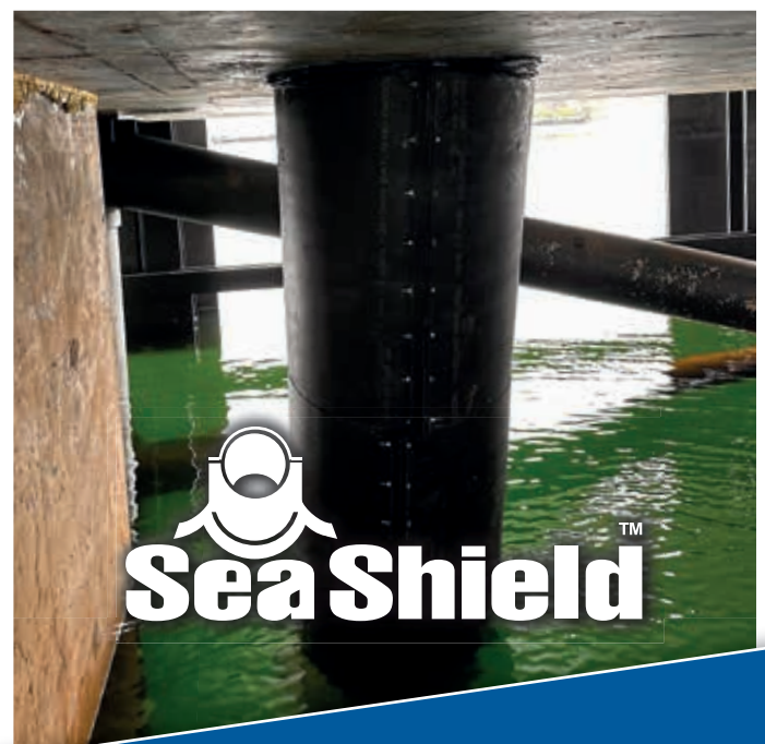
The complete Seashield 2000FD System protecting one of the piles.
