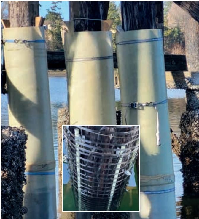
The SeaShield Jackets in place ready for the cavity fill of SeaShield 510 grout.
