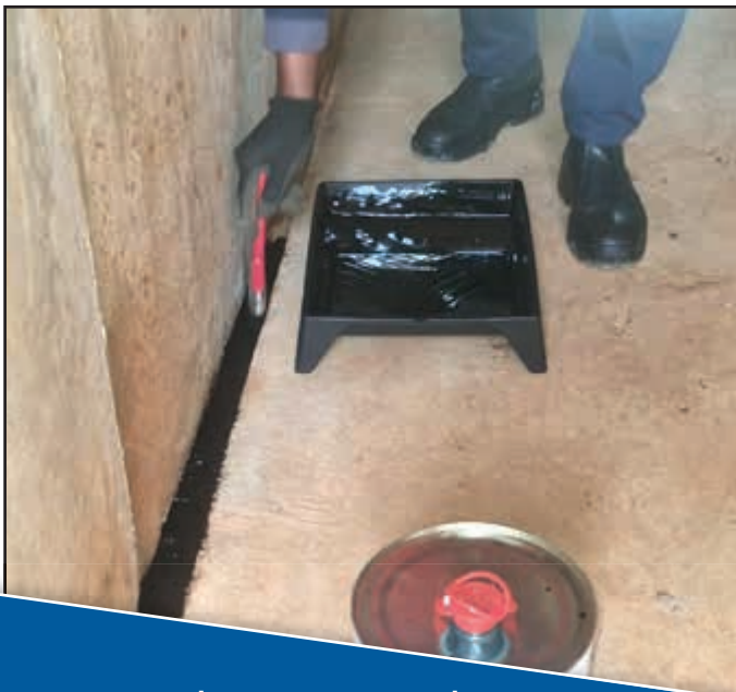
Denso Primer D™ and Denso™ Joint Sealer being applied on the inside of the culverts that have already been stacked.
