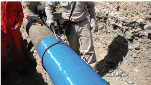
Following rehabilitation, the cathodic protection system was able to function normally again.
