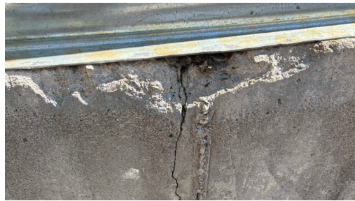
Deteriorating concrete foundation causing major structural issues at a silo facility.
